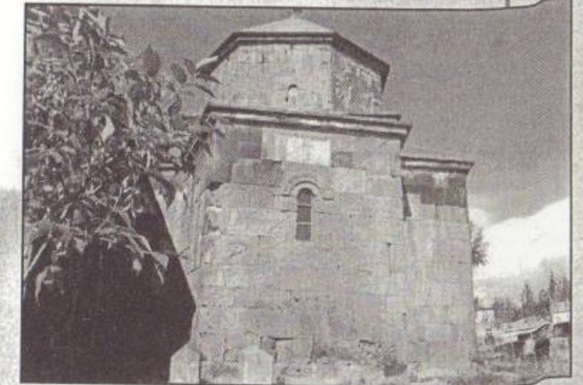
Gegharkunik marz, vil. Hatsarat, church St. Astvatsatsin (VII c.). Project director – Ashot Hovsepyan, head of the construction – Vazgen Ispiryan (reconstructed in 1982-1985).
