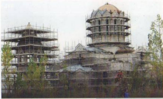
Image 7. Illegal "reconstruction" of Holy Saviour Ghazanchetsots Church of Shushi.
